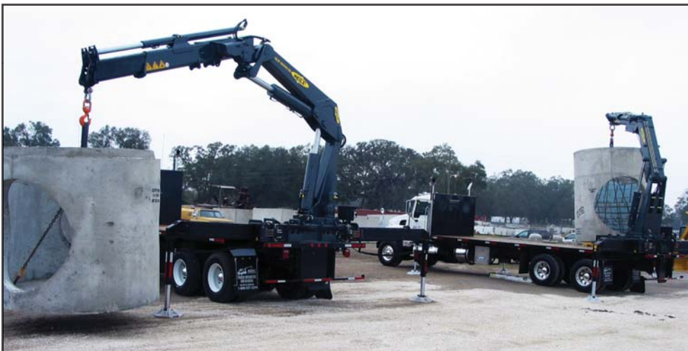
Unit requires a set up area for wide outriggers. A large enough area is not always available. Therefore more preparation for setting product is required.
